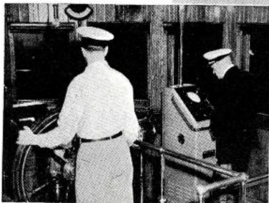
A GE parabolic reflector installed atop the pilot house of the "Ernest T. Weir." First Mate Gallagher and Captain Hartman are inspecting the installation.
