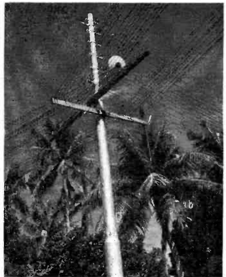
Photographic view showing elaborate pole line installations on New Caledonia.
