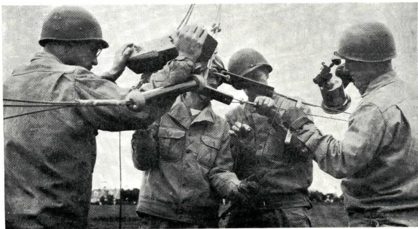
Soldering transmission wires on a rhombic antenna prior to hoisting on large telephone pole.
