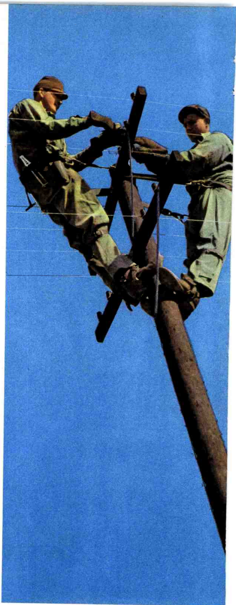
Crossarm being installed on pole by students of the long lines outside course, Ft. Monmouth.
